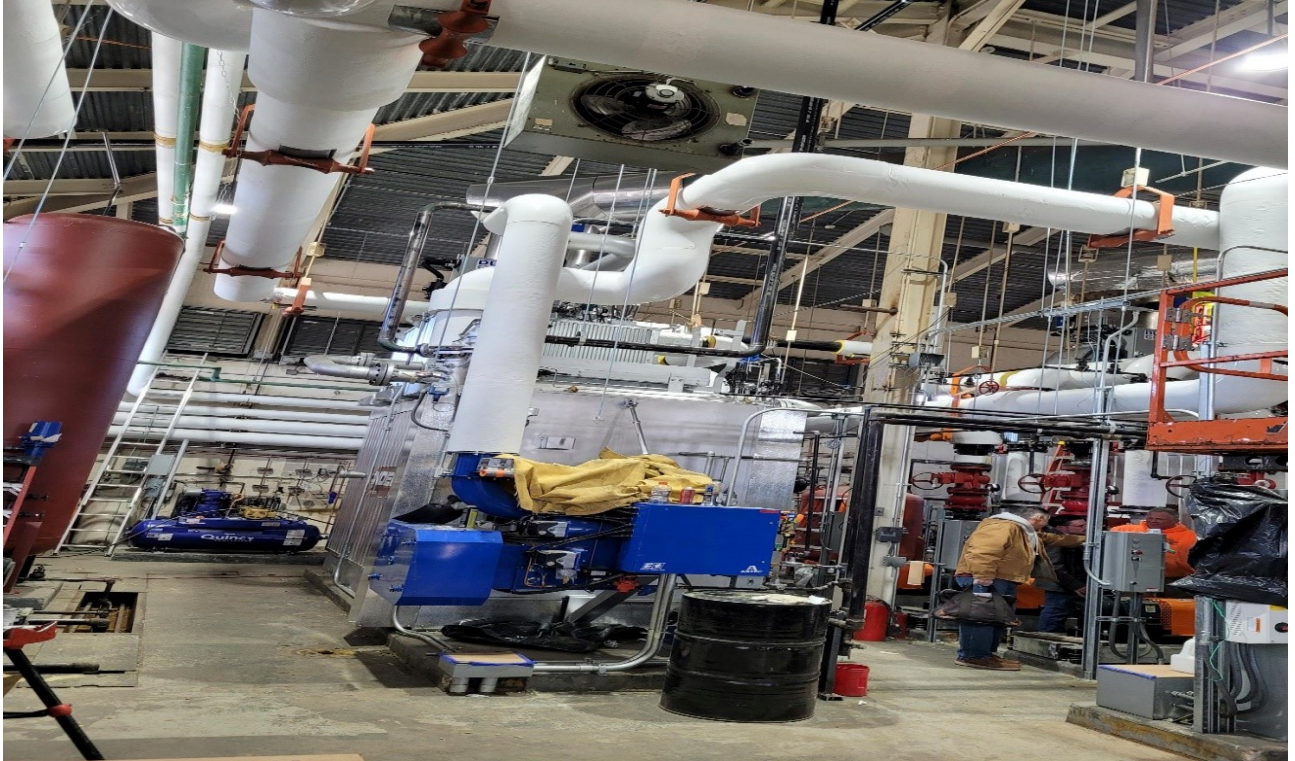
Eastern Campus Central Energy Plant New Boilers
